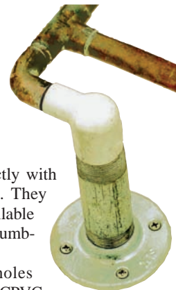
Figure 4 — Details of the galvanized steel pipe nipples mounted on floor flanges on the RV roof.
